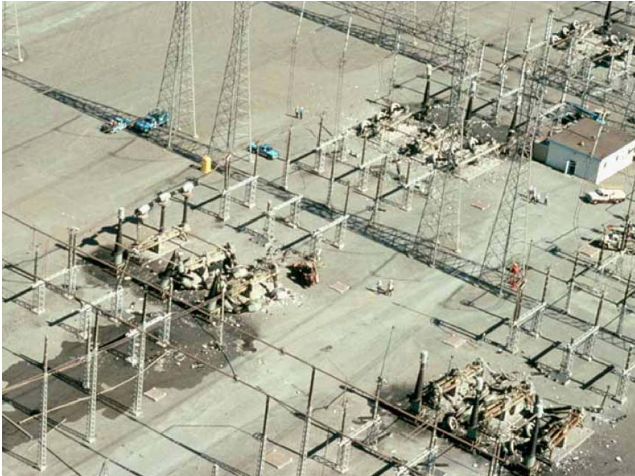
Figure 21: Moss Landing Switchyard after the Loma Prieta Earthquake, 1989 277
